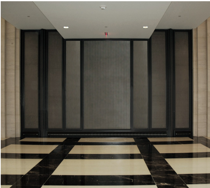
Center set of custom air intake louvers
