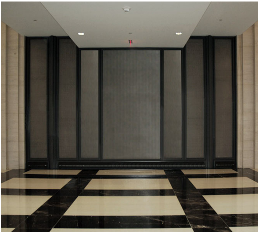
Center set of custom air intake louvers
